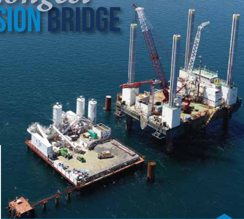
COMPLETE VIEW OF THE CHACAO CHANNEL, JACK UP BARGE AND SERVICE PLATFORM
