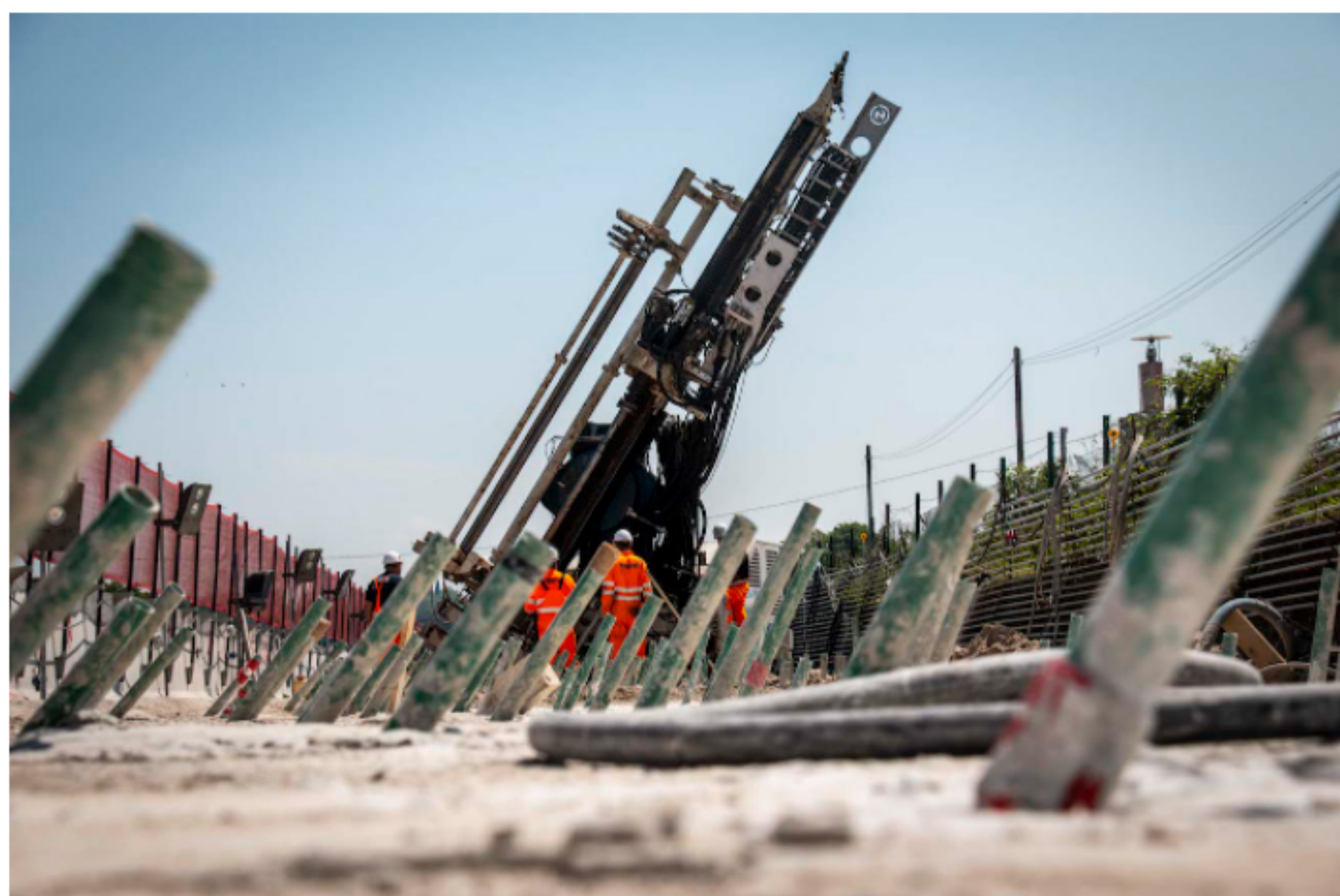
Sleeved pipes ready for cement and chemical grouting at the Lonato Tunnel site in Brescia, Italy (Photographs courtesy of Trevi)
