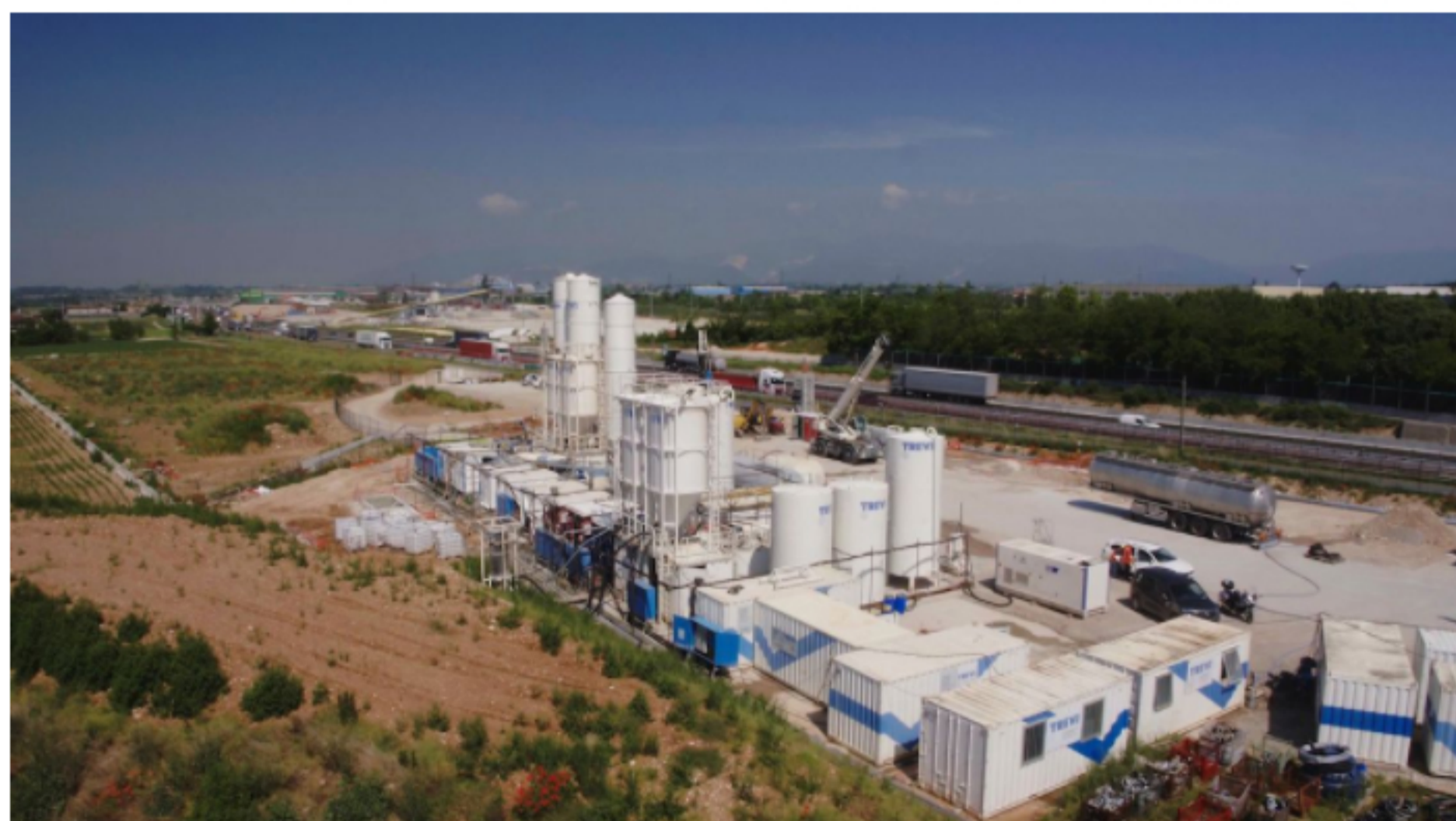
To complete the soil consolidation project, Trevi set up mixing plants for cement and silicate-based grout
